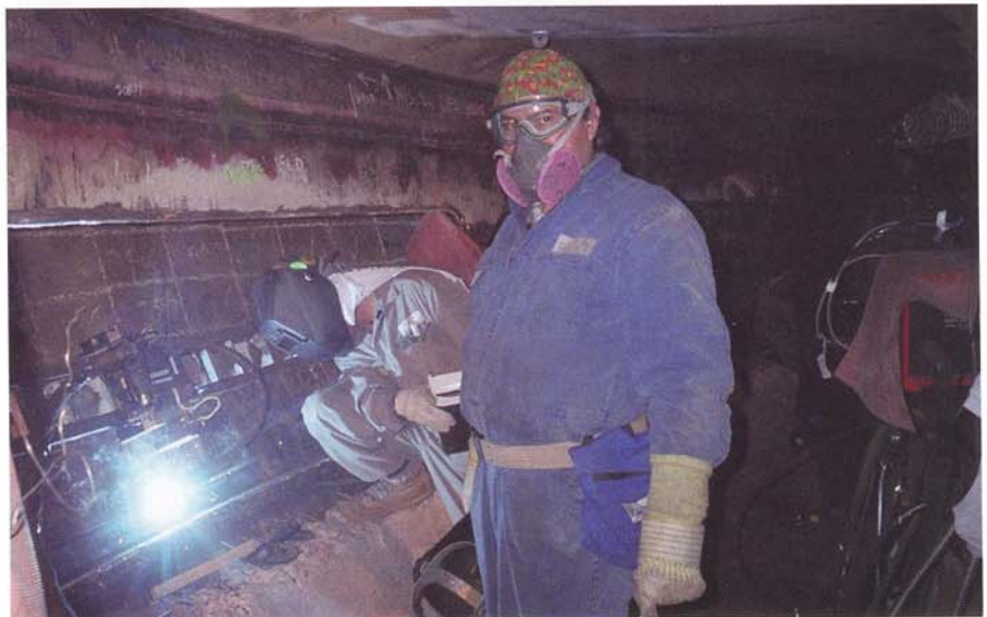
Fig. 3 — Nine-ft-wide windows were cut out of the inner skirt to allow access to the corroded steel shell.
